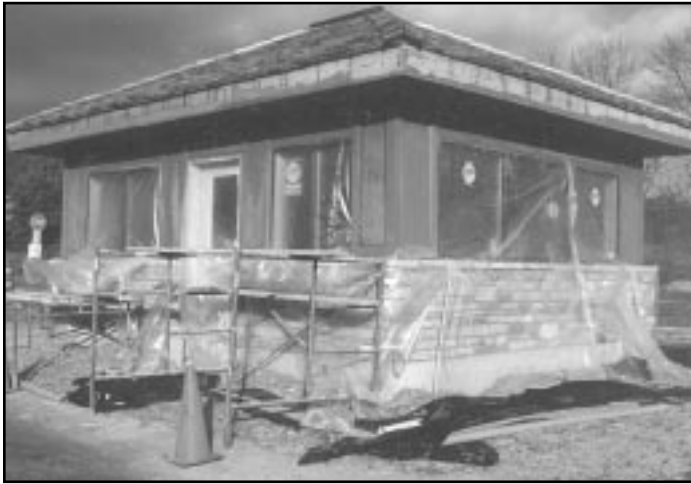
The SICenter went up quickly and was in use by February 1993, five months after ground-breaking.
